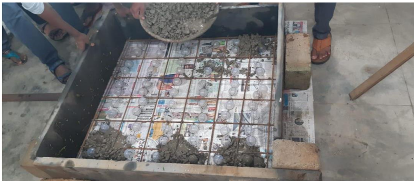
Figure 3.7 Placing of polypropylene balls in the centre of reinforcement & laying the concrete
