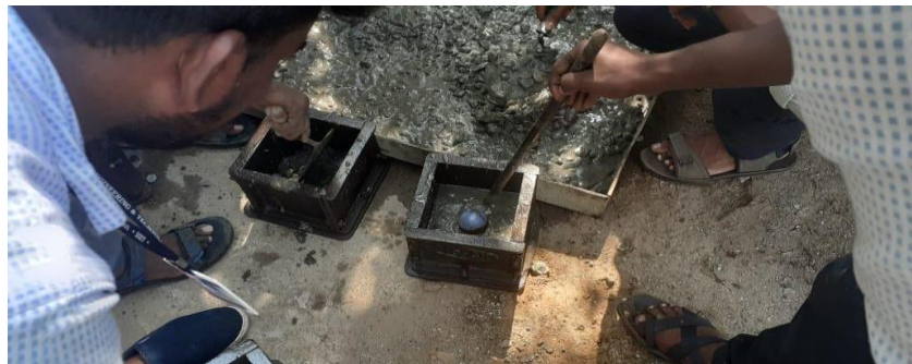
Figure3.2 Hand Tamping by using 50mm diameter of Tamping rod to compact the concrete.
